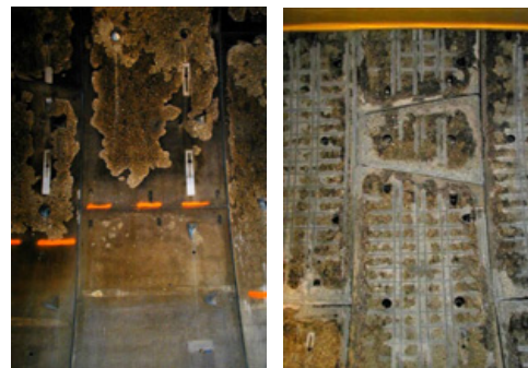
Figure 6a, Figure 6b: damaged areas on concrete liners
